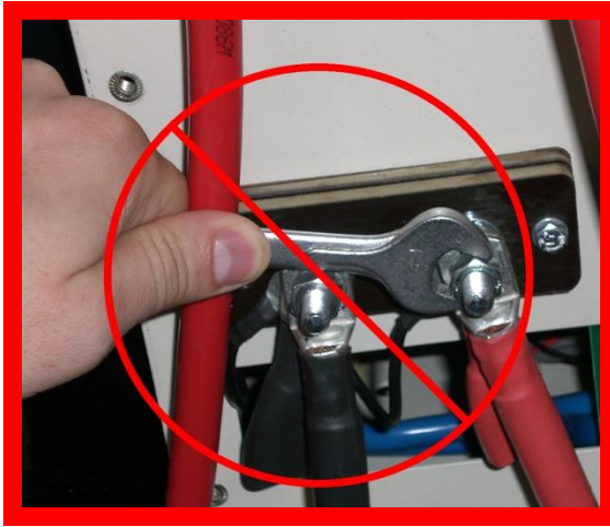
Figure 24: Danger of Short Circuits when using an Un-insulated Spanner to Connect/Disconnect Batteries
